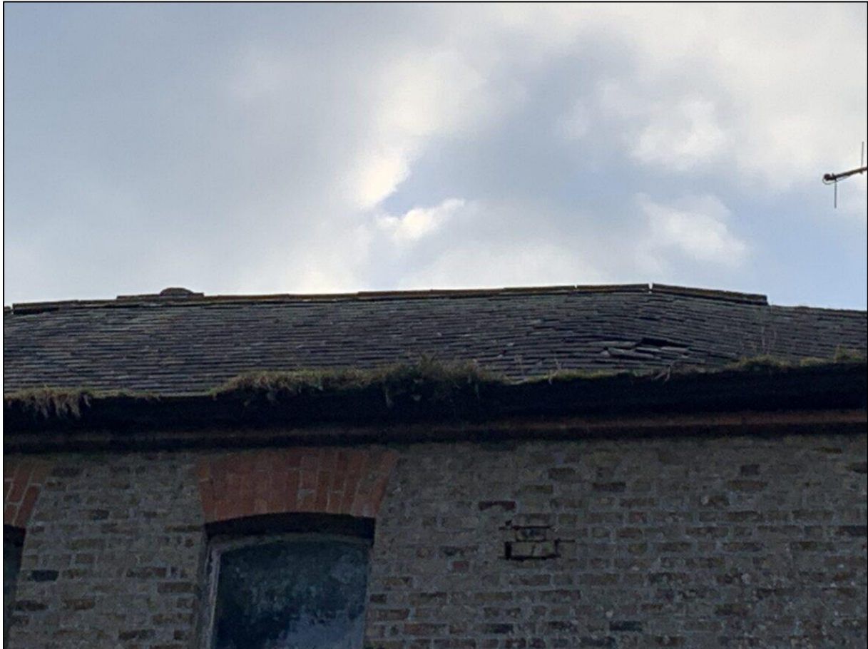
Plate 3-1: Loose roof slates on the coach house
