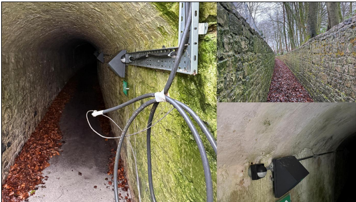
Figure 5: servant's entrance tunnel emergency lighting is in place in the tunnel, but was not extended along the walkway (upper right picture)
