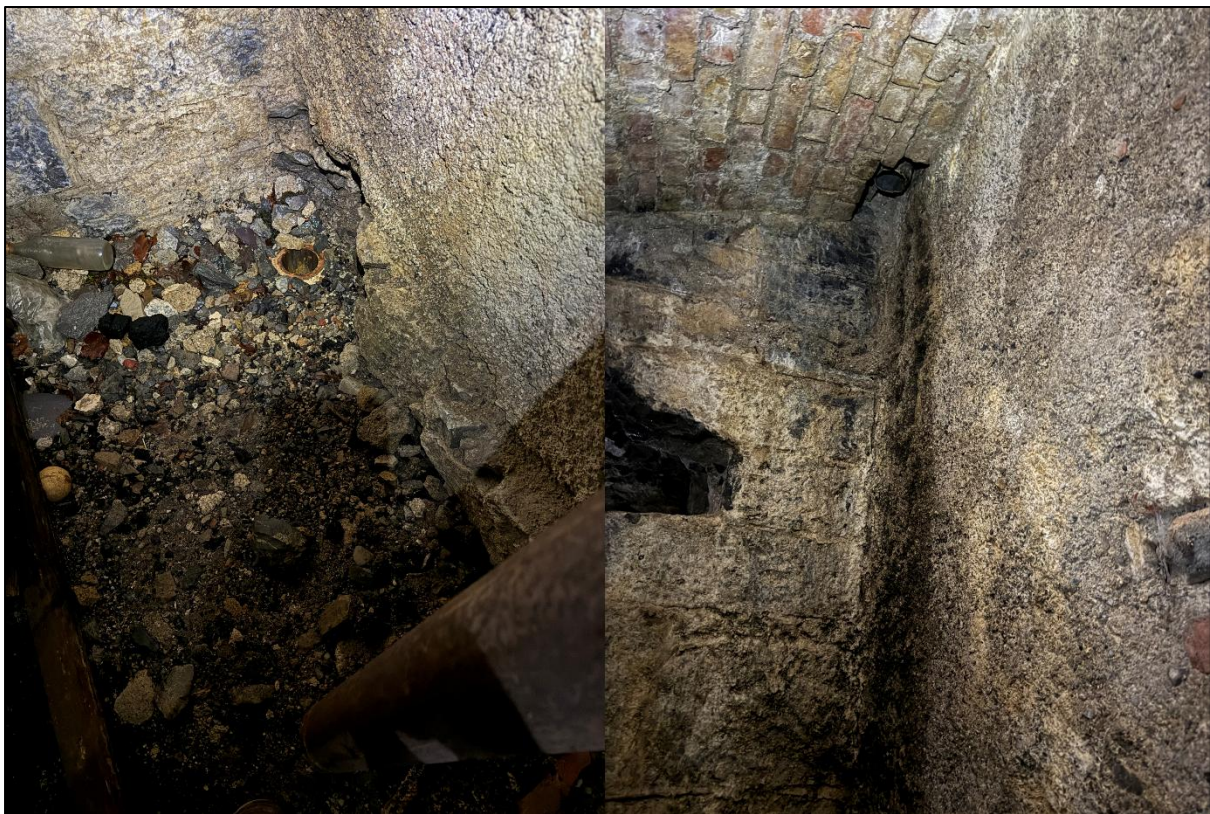
Figure 6: Section of missing down pipe and dampness on wall where pipe requires reinstating
