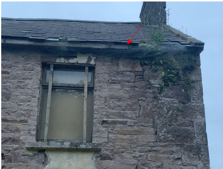
Plate 3-4: Gap under roof tiles
