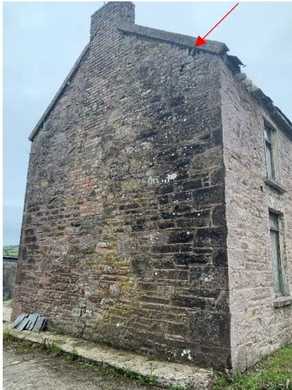
Plate 3-3: Gaps between stonework
