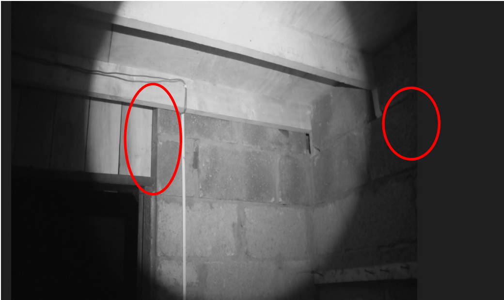
Plate 4-6: Location of cavities within shed (structure 3)
