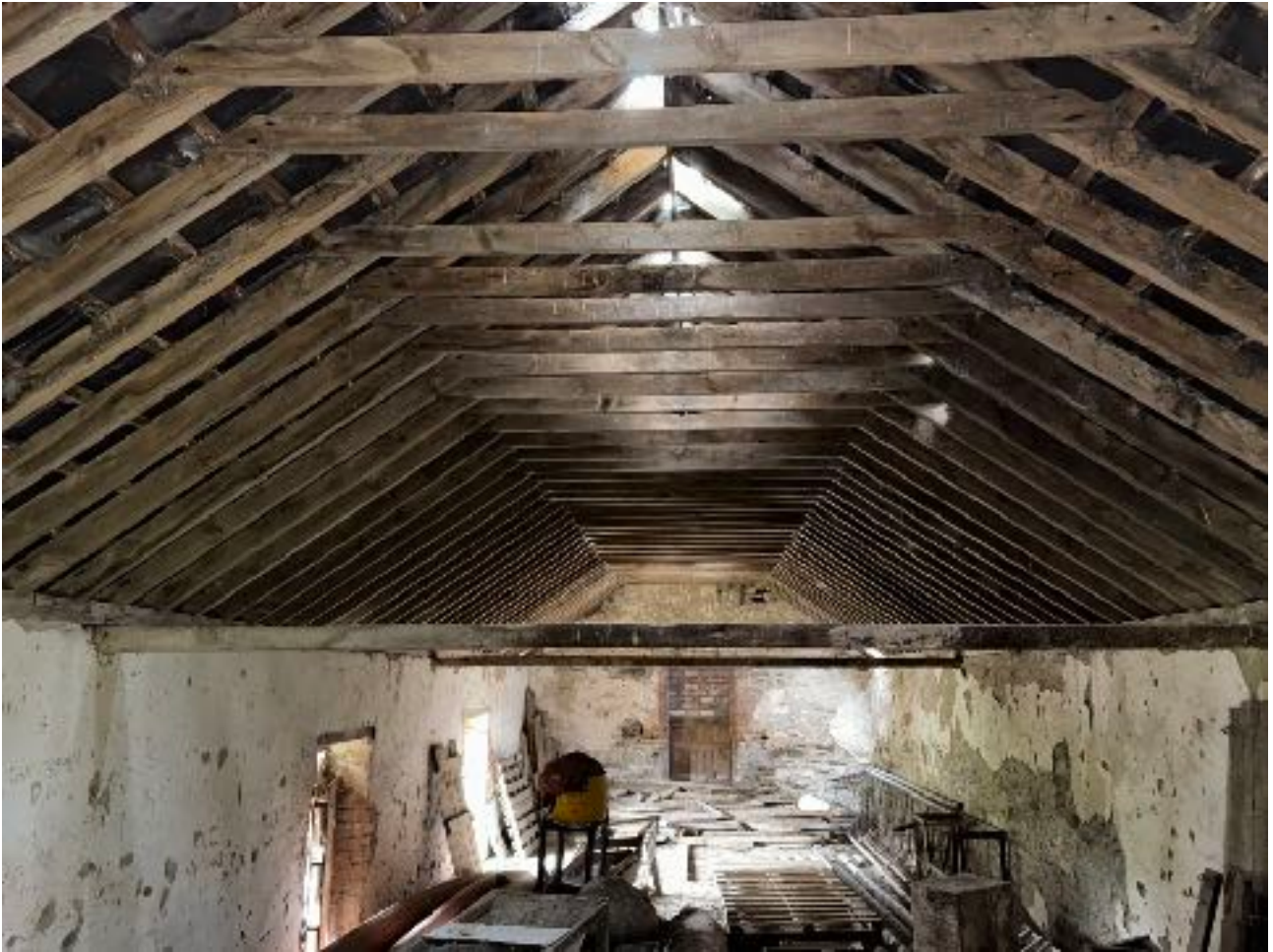
Inside upstairs of Lamberton's barn looking towards southern gable end and leisler roost. Note the lack of cobwebs.
