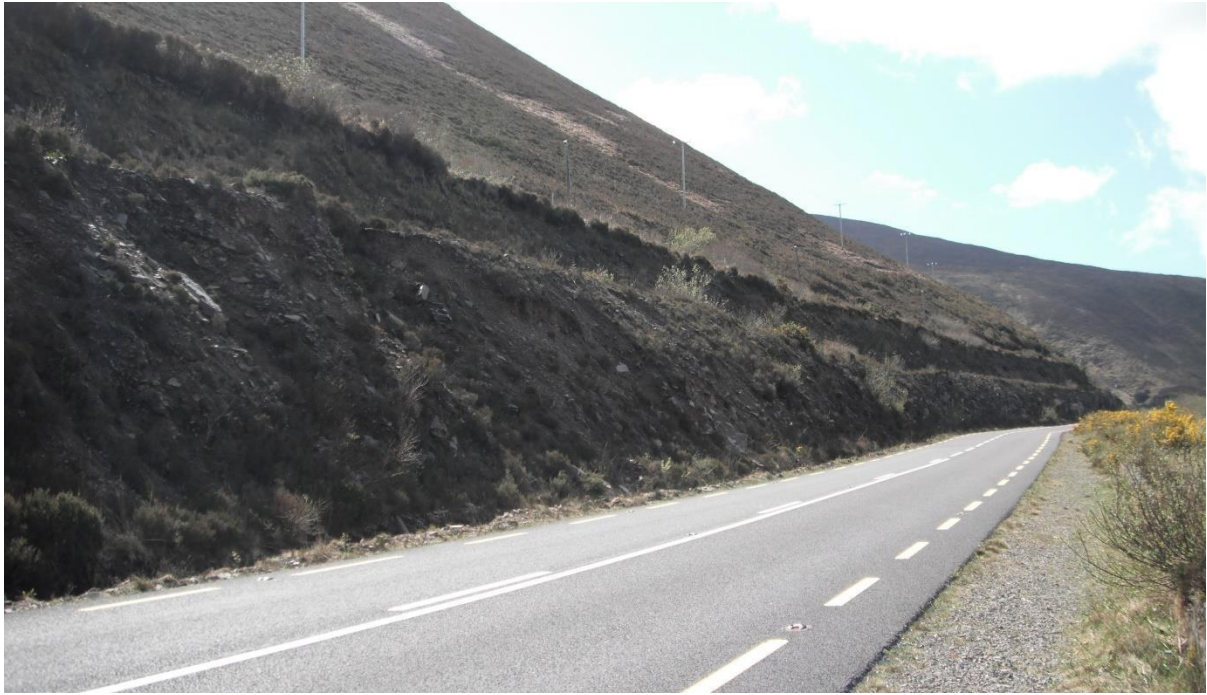
Plate 11: View west (towards Drung Hill Tunnels) showing N70 and existing profile where gabions will be constructed.
